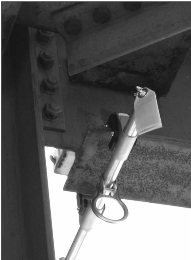
Fig. 16. Danger: Beam clamp near coped end
