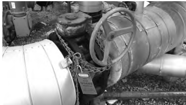
Figure 33-5: Close, Chain, Lock, and Tag Pipe Valves
